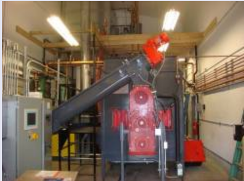
3 MMBtuh Hot Water 25% Char+Ash
